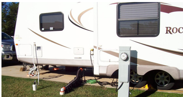
FIGURE 22 Utility Hook-Ups RVs are designed to be self-sufficient for short periods of time. But, for longer stays they can be plugged in to standard domestic utilities. In this image the RV is connected to water, sewer, and electrical.
