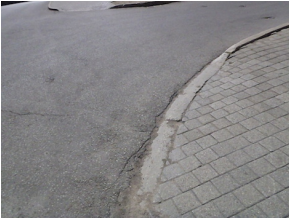
WP057 – Curb cut with uneven transition.
