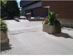
WP061 – Uneven transition between surfaces.
