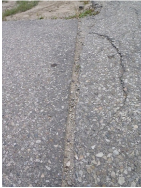
WP013 – Seam in pavement with 2.54cm width.
