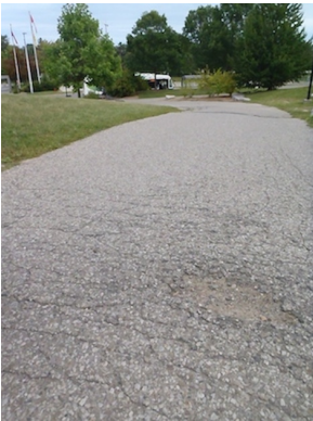
WP014 – Broken pavement with 2.54cm hole in center of walkway. Width of hole was 43.18cm wide and 22.86cm in length.
