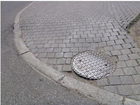
WP058 – Curb cut with uneven transition. Concrete bordered by broken pavers on walkway side. Manhole protrudes above grade with missing pavers between the cover and concrete of the curb cut.
