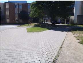
WP059a – Curb cut with uneven transition.
