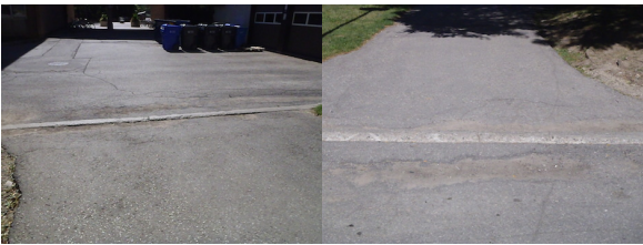
WP059 – Curb cut (on alternate walkway) had protruding concrete. Areas on each side of concrete are below grade. Curb cut with uneven transition.
