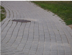
WP064 – Protruding utilities cover created transition and affected placement of pavers.
