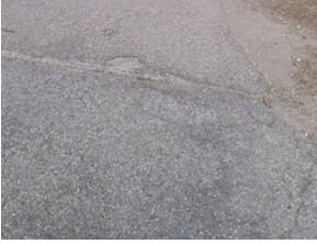
WP011a – Hole in pavement along seam in walkway.
