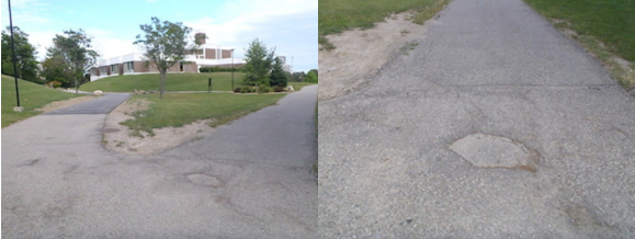
WP012 – Seam in pavement width 137.16cm wide with whole in surface.
