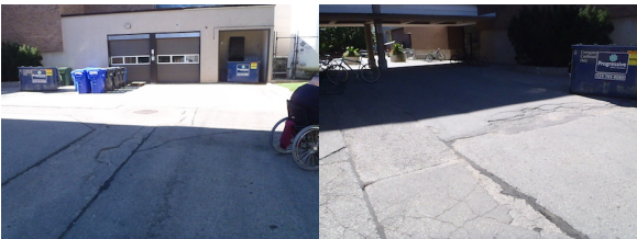
WP060 – Large area of pavement with multiple surface issues. Pavement is fragmented or missing creating an inconsistent surface.
