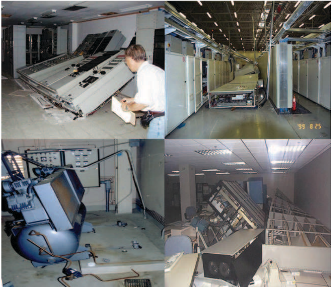
Figure 1.2 Damage of secondary systems in earthquake events
