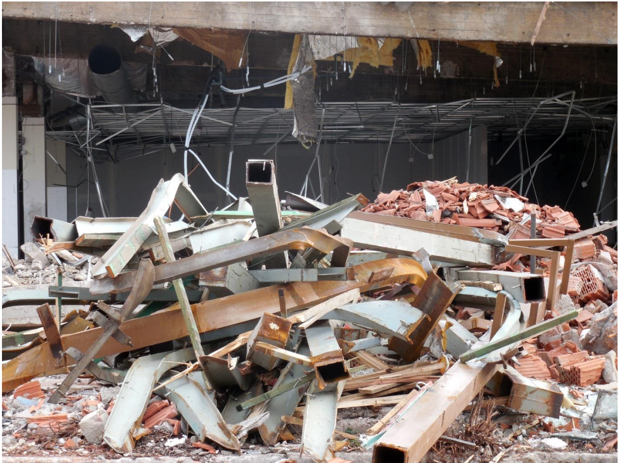
Figure 2-3: Typical damage to steel members sustained during demolition
