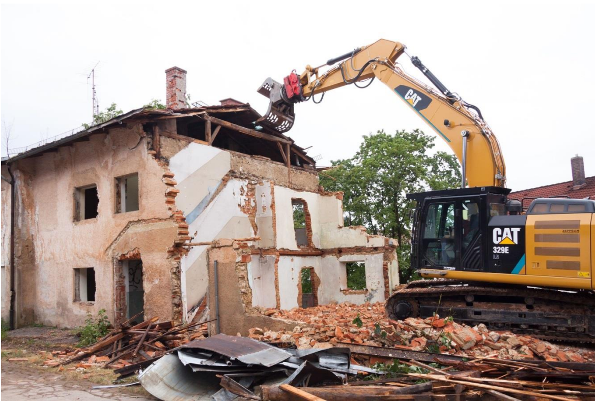
Figure 5-4: Excavator with hydraulic grapple being used for the demolition of a structure
