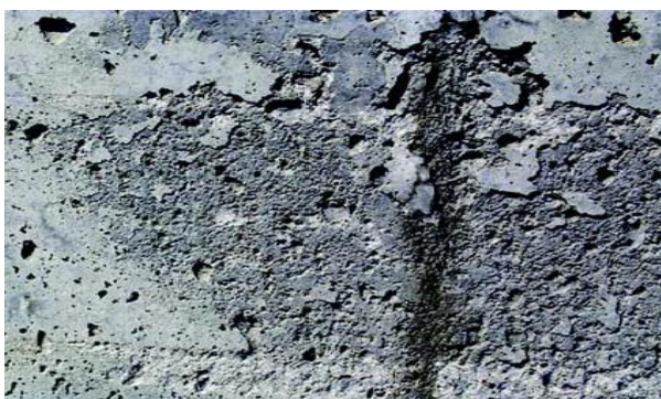
Figure 2-4: Example of medium spalling of a concrete surface (ACI 201.1R-08)
