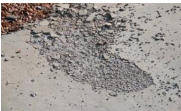
Figure 2-5: Example of concrete flaking or spalling ( http://concretetoolreviews.com )
