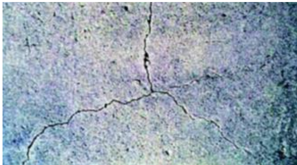
Figure 2-3: Example of shrinkage cracking (ACI 201.1R-08)
