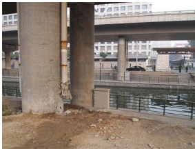
Figure 09.16.b: Decaying infrastructure surrounding the project in contrast to the new construction of Linked Hybrid in the distance.
