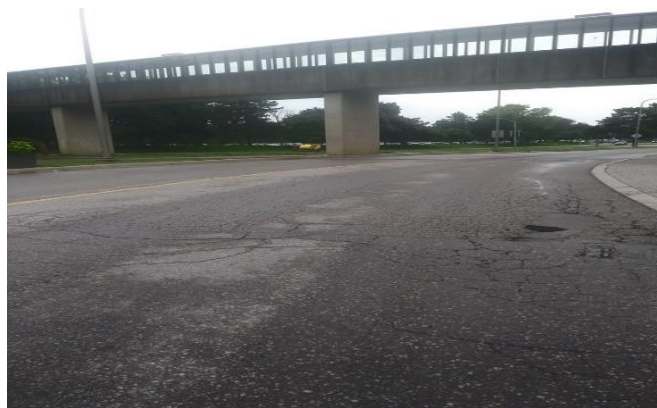
Figure 2-7 Fatigued cracking in pavement (Waterloo, Canada)
