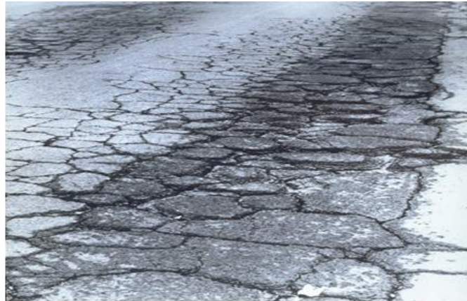
Figure 2-8 Fatigued cracking pavement “alligator cracking” [28]
