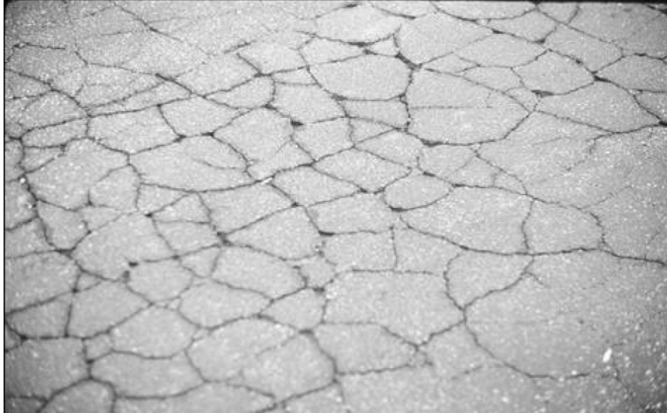
Figure 2 - 5: Fatigue (alligator) cracking (Miller et al., 1993)
