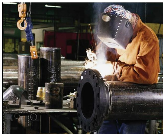
Figure 1-1: Welding of cover pass on a joint in Industrial Piping using SMAW [4]
