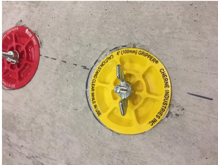
Figure 3.9: Photo of Expansion Plug Used to Seal Core Holes After Core was Removed
