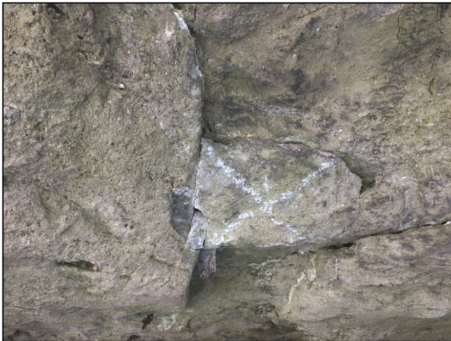
Figure 6. A loose block ‘X-d’ out.
