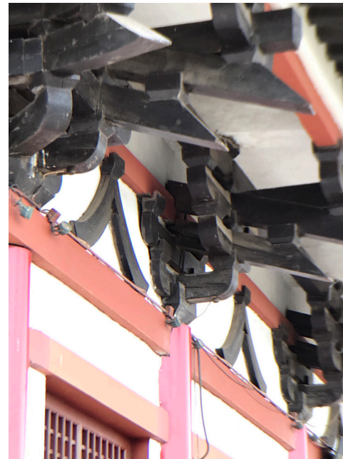
Figure 2.56 Bracket detaching from the concrete wall, Zhong-hua Temple, Shenyang, Liaoning, China
