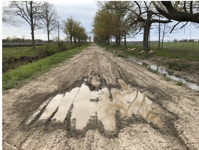
Figure 2-6 Damaged road due to rainfall and loading effects (Picture was taken in Niagara, 2017)
