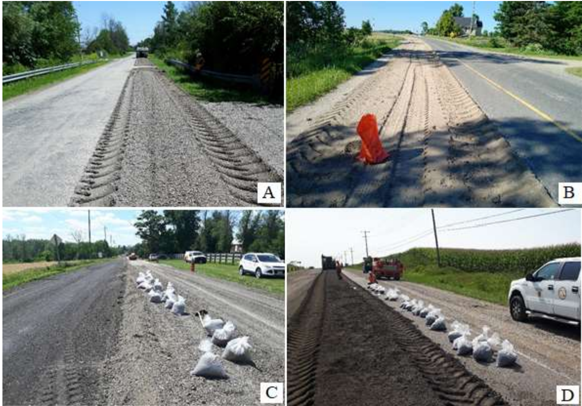
Figure 3.2 Full-depth reclamation projects A) Niagara-on-the- Lake, B) Bruce County, C) Kossuth, D) Nafziger
