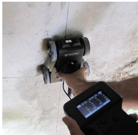
Figure 7.9. Recording the rebar's magnetic data from the surface of concrete using PMI scanner (blue line shows the rebar's orientation).
