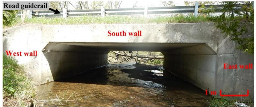
Figure 7.3. Culvert C072, with walls' names (North wall is on the other side of the road and cannot be seen in this picture).
