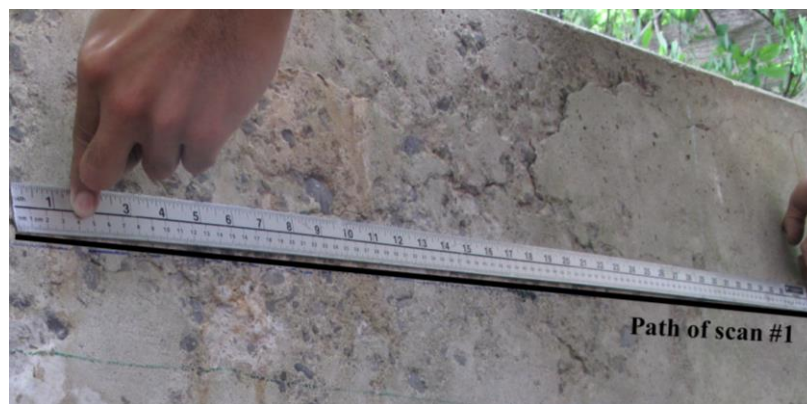
Figure 7.14. Concrete conditions from 400 cm to 500 cm (from the West wall) in the path of scan #1.
