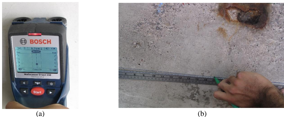
Figure 7.7. Pre-inspection activities before recording the magnetic data: (a) Locating rebars using a rebar detector; (b) Marking rebar paths using a permanent marker.
