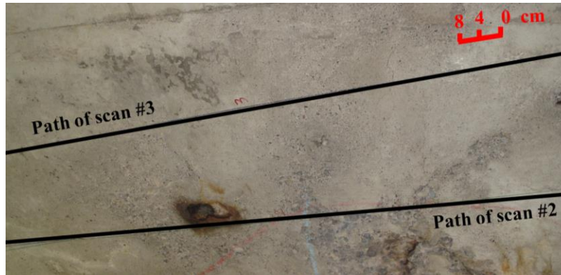
Figure 7.15. Concrete conditions from 100 cm to 200 cm (from the West wall) in the path of scans #2 and #3.
