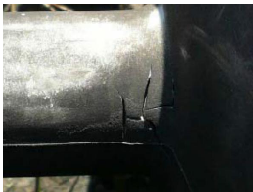
Figure 2.12. Deterioration on the aged silicone rubber insulator [44].
