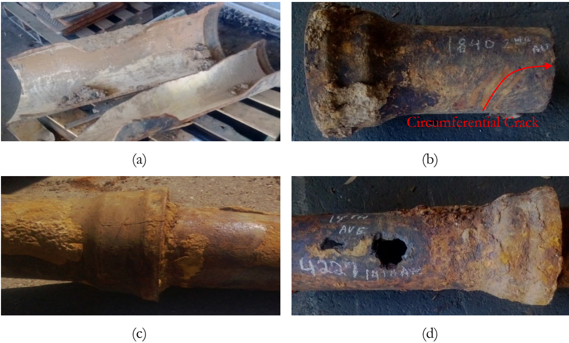
Figure 2.3: Different modes of failure (a) longitudinal failure (b) circumferential failure (c) split bell (d) corrosion holes (from pipe fracture data, The City of Sacramento).
