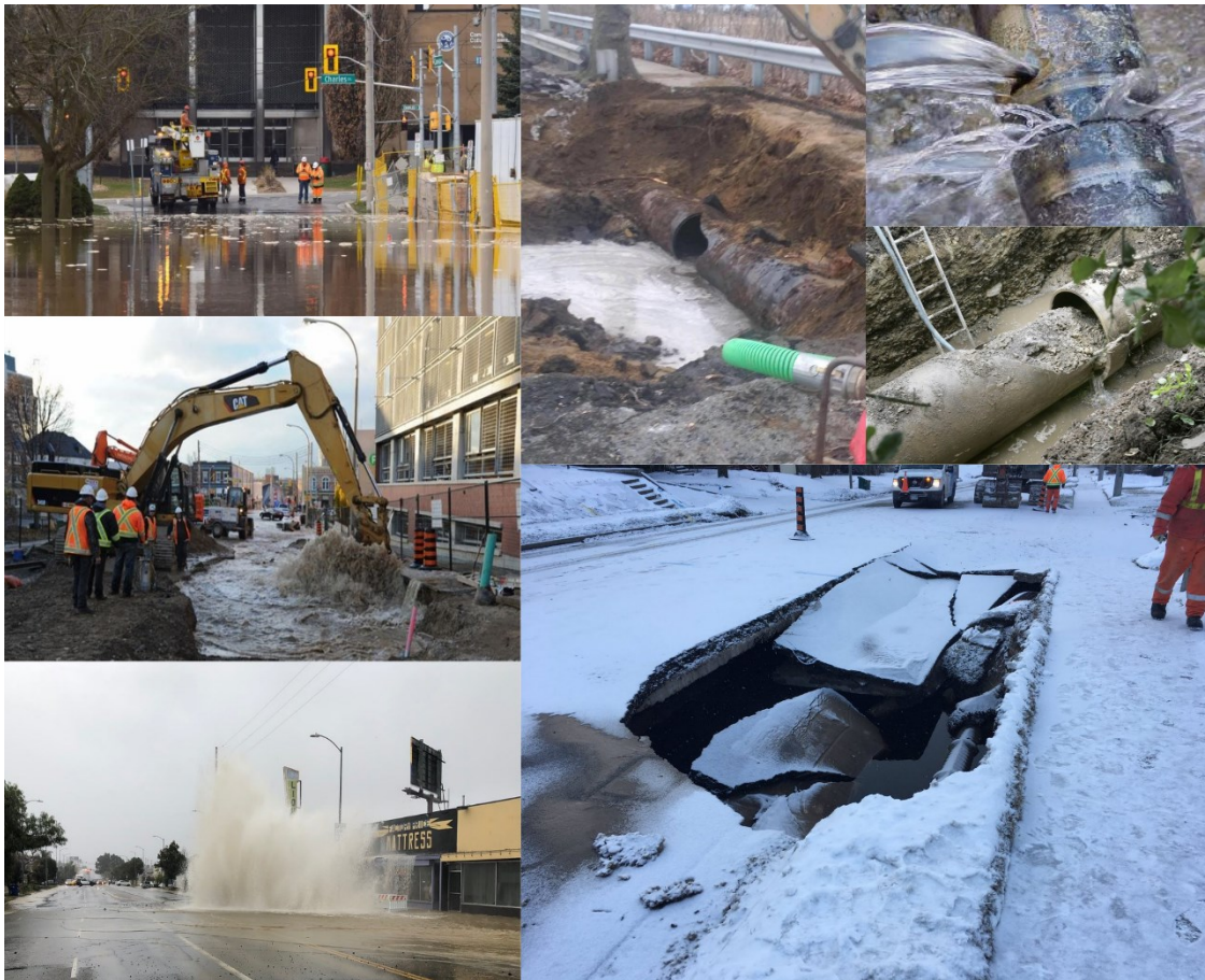
Figure 1.1: Water main failures 1 .
