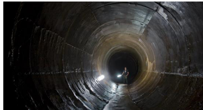
Fig. 2.2 The Spadina Storm Trunk Sewer built to redirect the Castle Frank Brook in Toronto.
