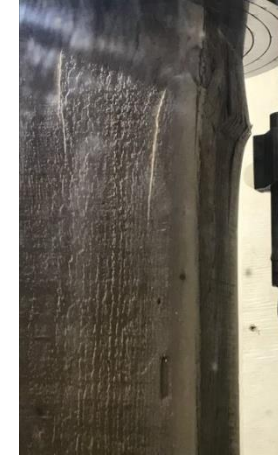
ii) Face Splitting Off
