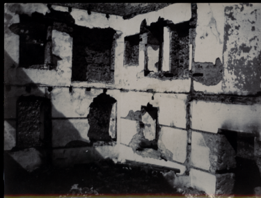
52.8 Interior of Destroyed American Girls' High School in Kessab, K1988.011.169
