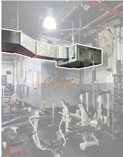
unappealing ceilings with hvac clutter
