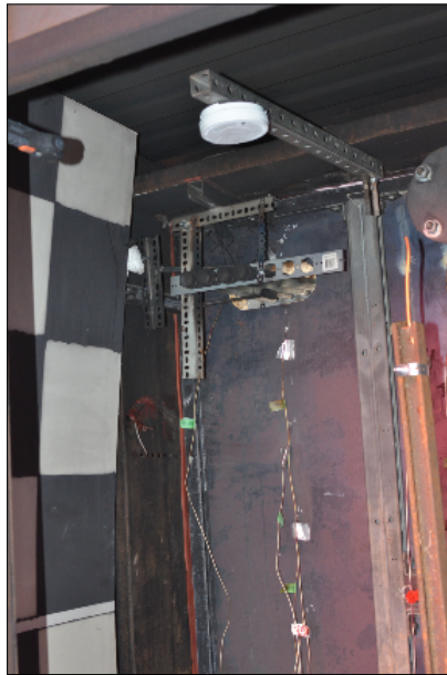
Figure 3.12: Photo showing actual pipe and pipe hanger configuration at opening from the rear view
