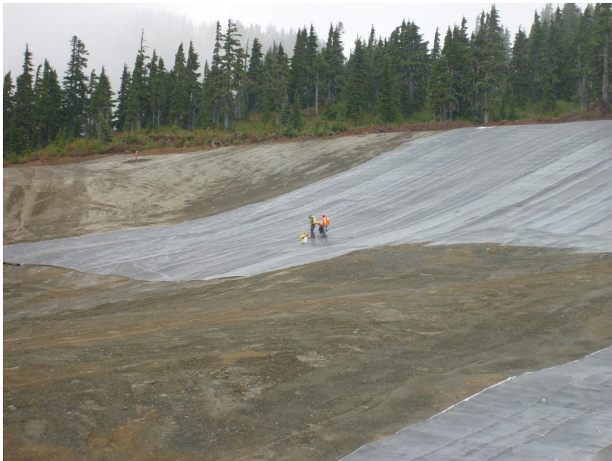
Fig. 4.17 The installation of the bituminous membrane cap. (Source: Photo used with permission from the Tsolum River Restoration Society, BC)
