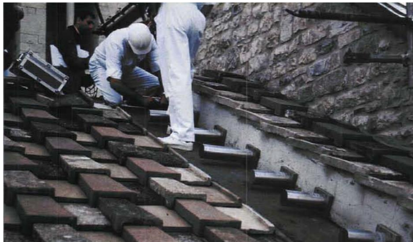
Figure 2.19: Cylinders Containing SMADs to Connect the Tympanum to the Roof in the Basilica St Francis (Crocì, 2001)
