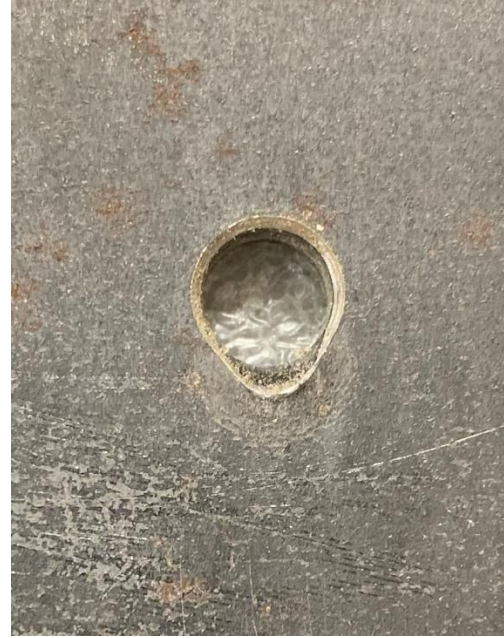
b) Non-Reusable Steel Plate Damage
