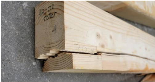
(c) Close-up of damage for R1-02
