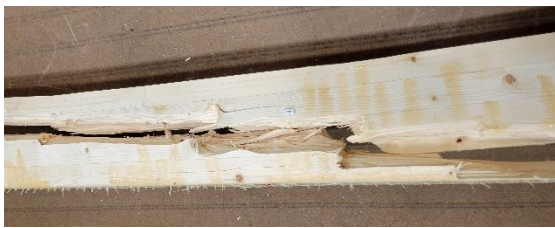
(a) Close-up of damage for R2-01
