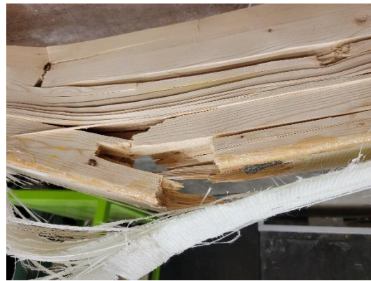
(c) Close-up of damage for R12-02
