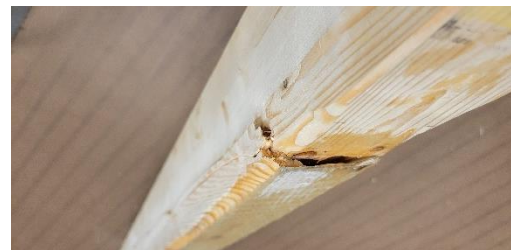
(b) Close-up of damage for R1-02
