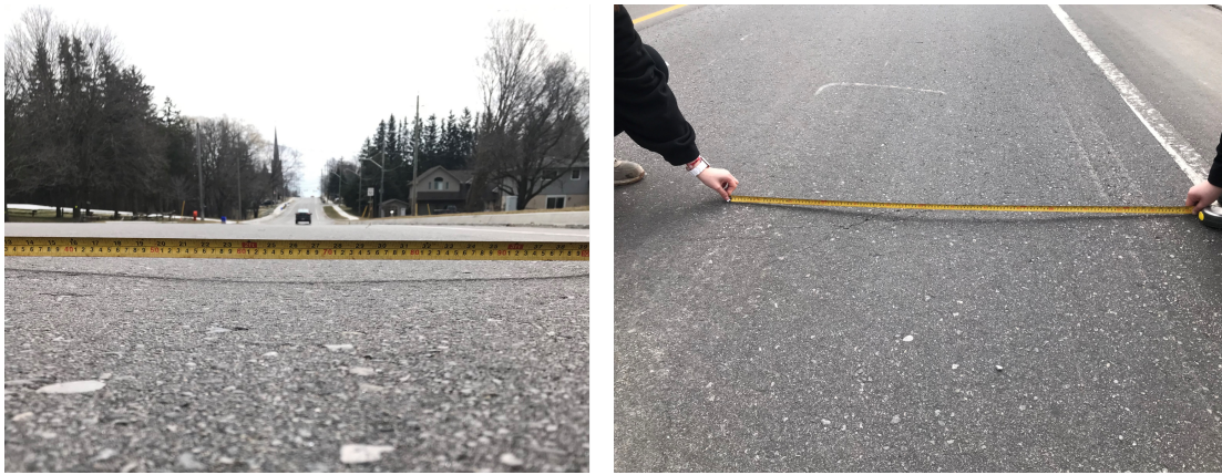
Figure 2.2: Permanent deformation (rutting) - The pictures were taken by Abimbola Grace Oyeyi
