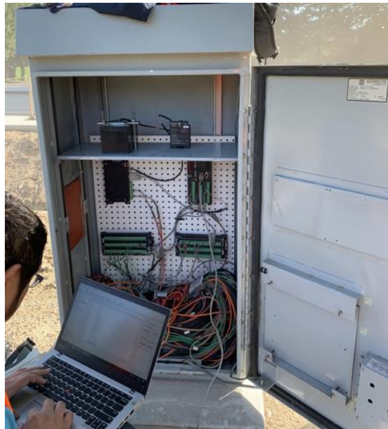
Figure 2-12 Data acquisition and control system panel
