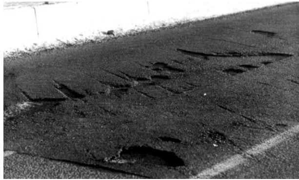
Figure 7 After the first snowplough Norwegian trial section near the joint with the hard asphalt surface
