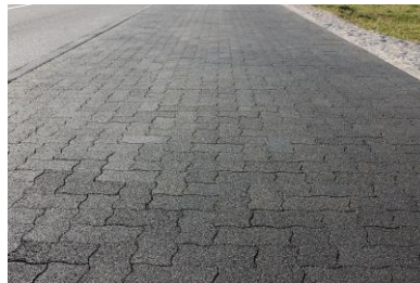
(e) Test track in Nova Gorica, Slovenia, built in December 2014 (length 20m). This poroelastic block pavement is made of PERS tiles glued onto cement concrete blocks.
