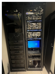
(e) Control Room
