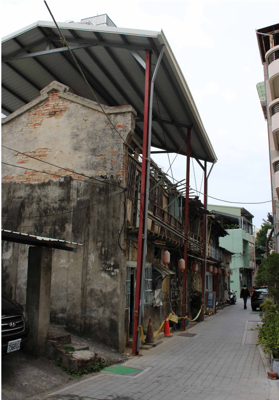
Fig. 2.42 Some worn-down Japanese streethouses constructed of wood, with Minnan-style masonry walls acting as structural support. The first floors of these houses are still occupied by residents.
