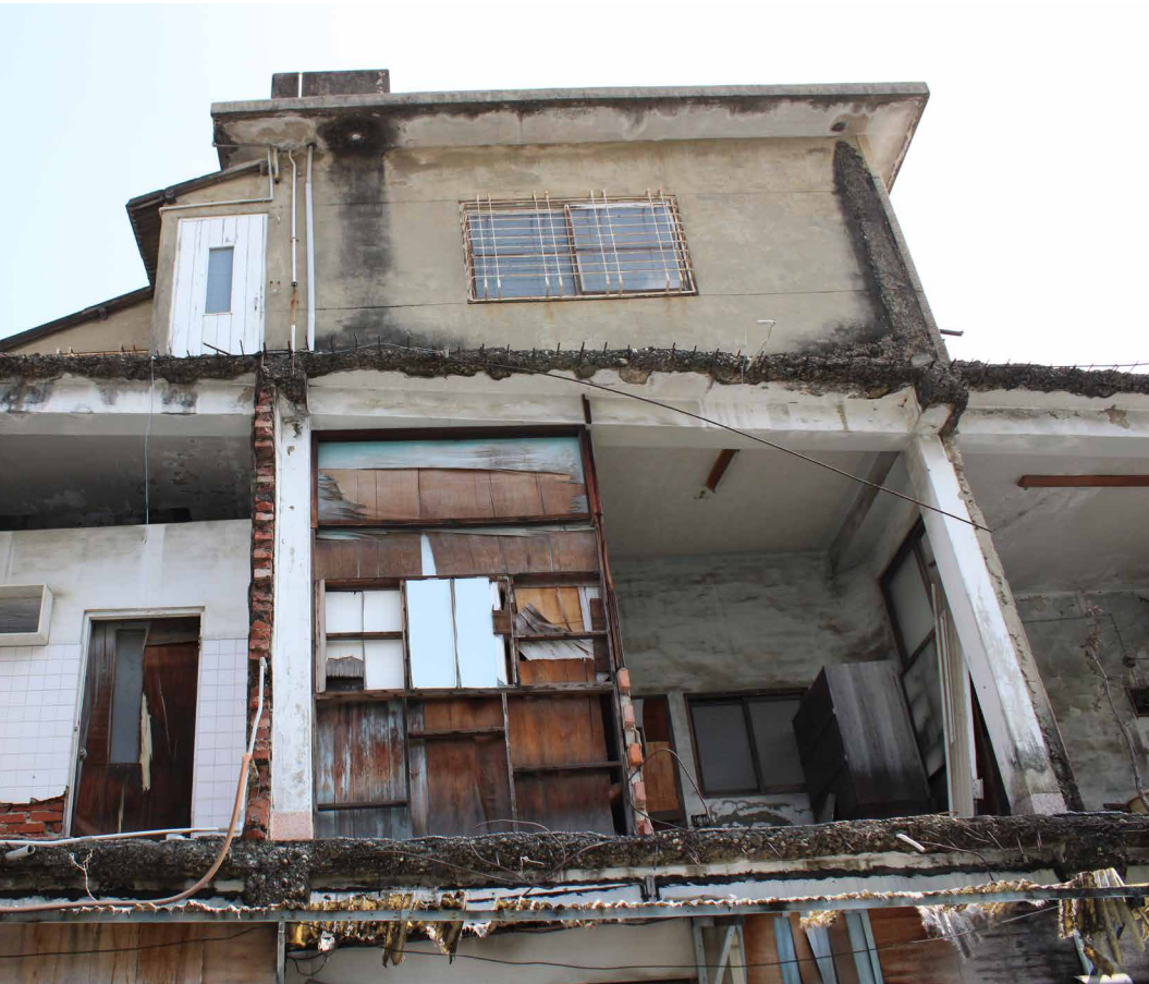
s exterior walls missing. Much of the house is actually left intact, allowing passerby inal masonry structure on the left side of the home (which was likely a kitchen the ete walls on the right side of the home which was likely added on later.
