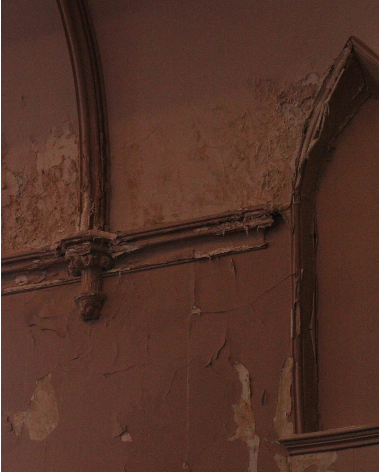
Fig. 4.18 The ceiling and wall along the south wall have experienced extensive damage from a roof leak, posing structural concerns.
