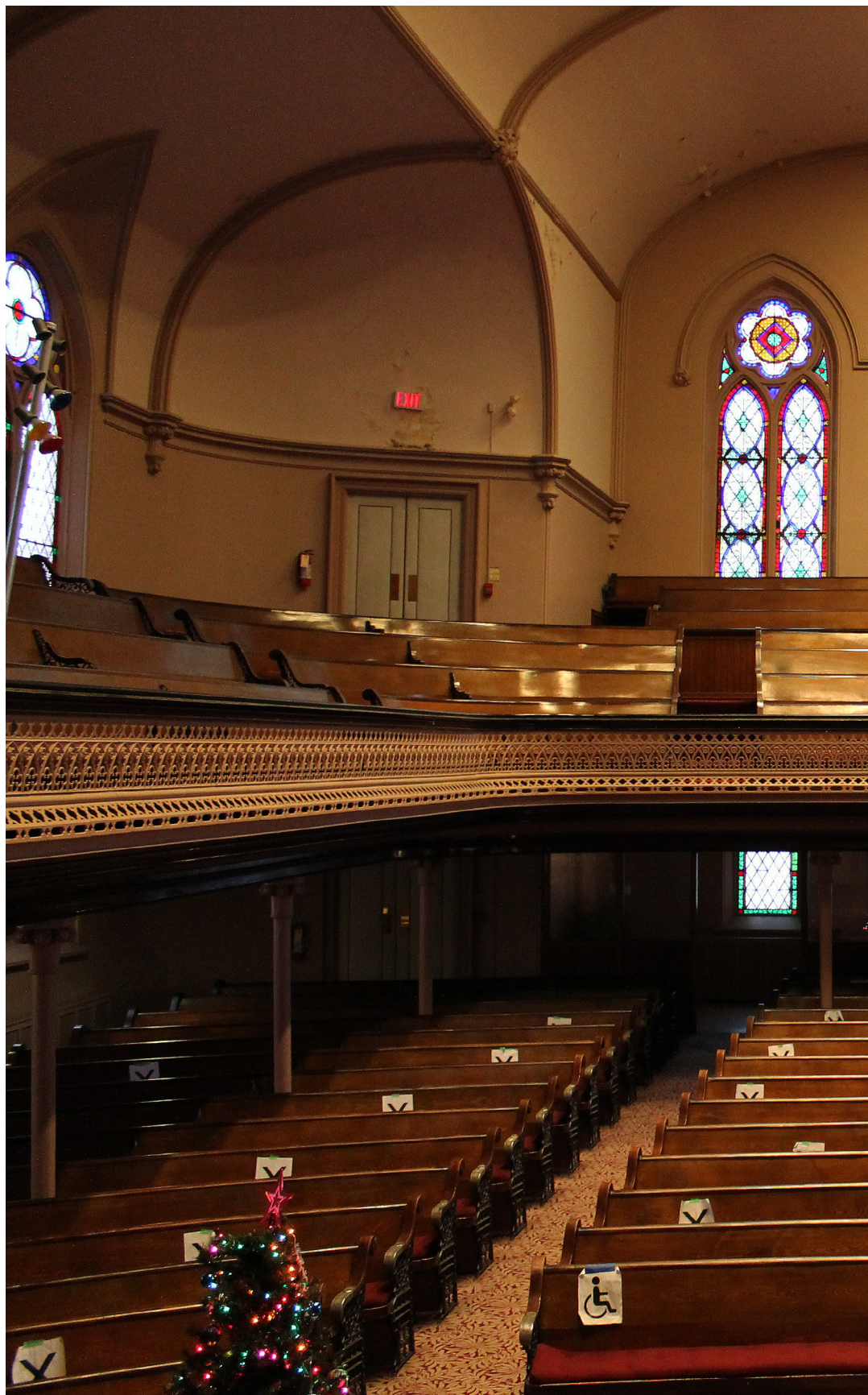
Fig. 4.21 More signs of water damage along the ceiling and wall towards the front of the church building.
