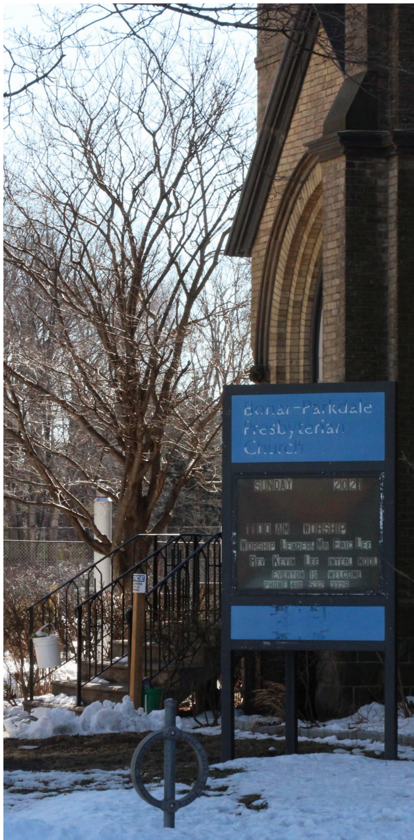
Fig. 4.11 In the winter of 2023, the church billboard has not been updated since 2021. Plastic buckets are placed at the ends of the front stair treads and railings due to the frequent littering and drug paraphernalia that is left behind.
