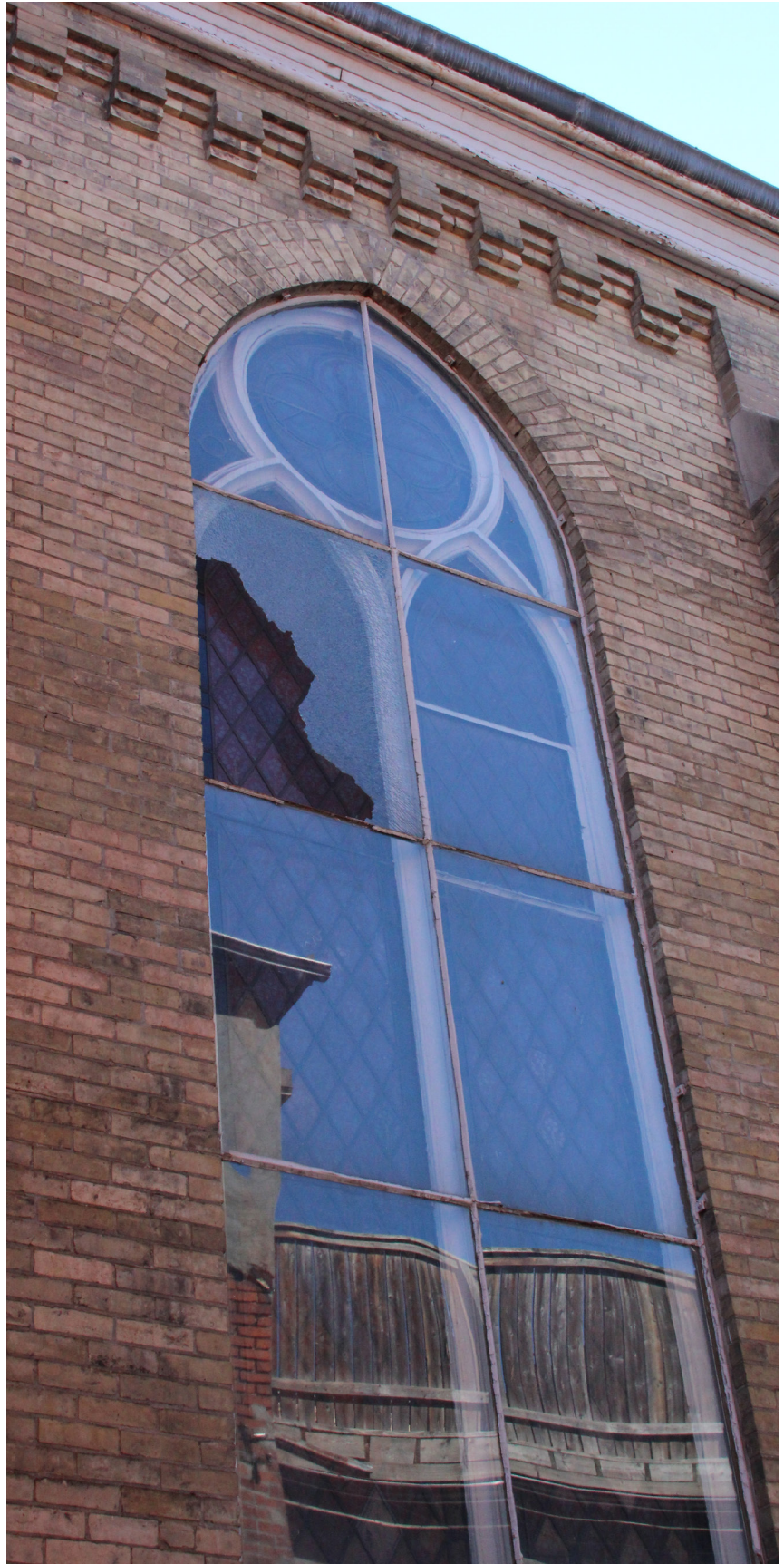
Fig. 4.14 Two of two glass panes on the north facade of the church that is partially broken.
