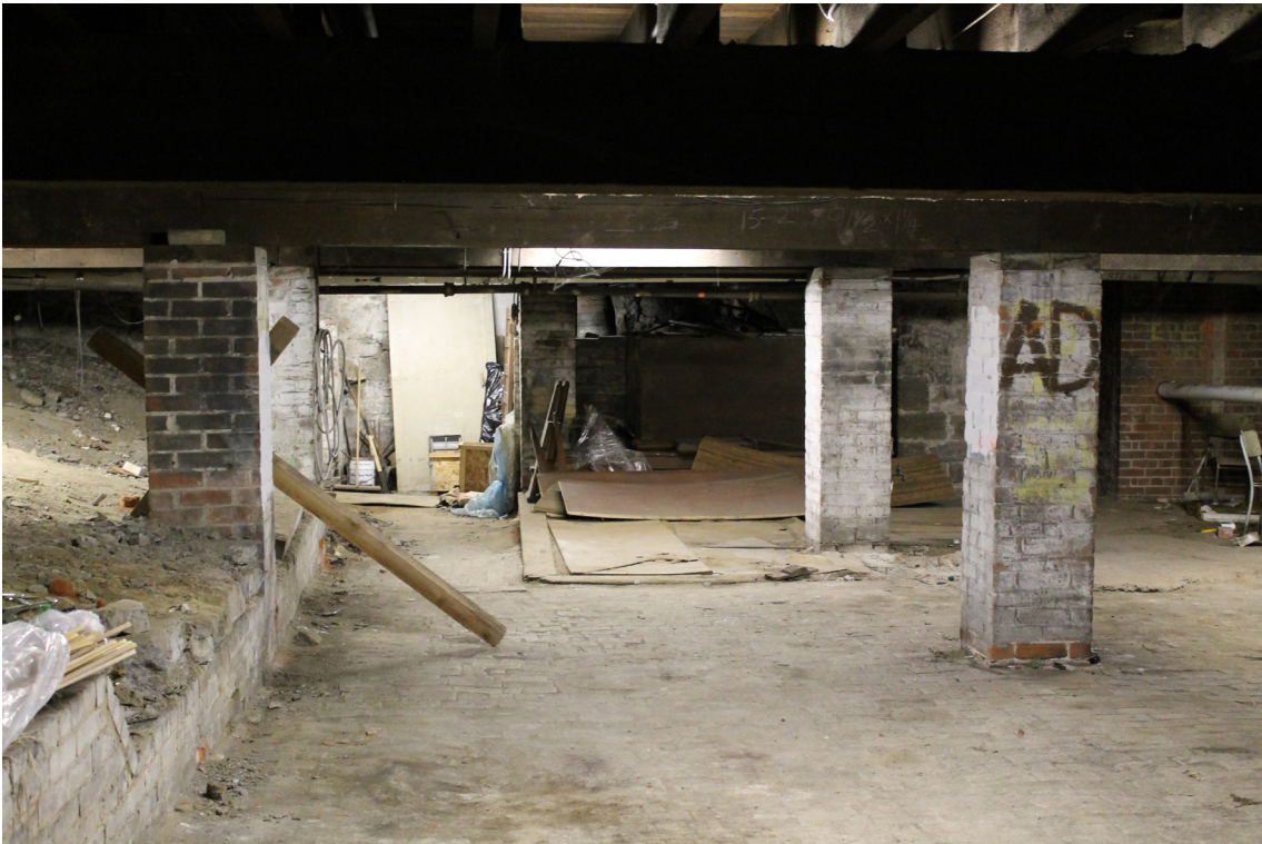
Fig. 4.19 The church basement is used for miscellaneous storage with access to some of the building's service equipment.
