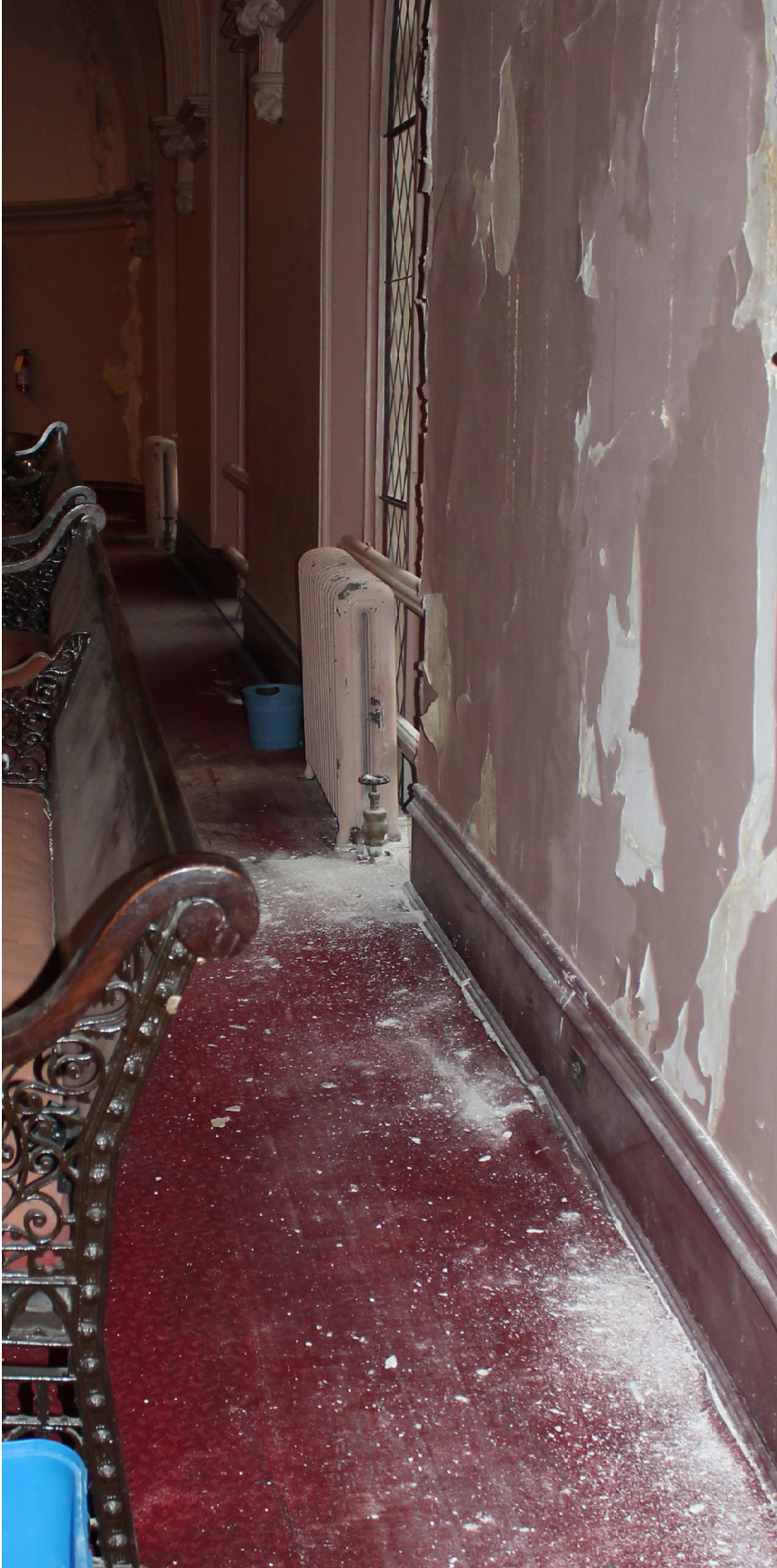
Fig. 4.17 Dust from water-damaged drywall collects on the floor of the sanctuary gallery. Buckets collect water during rainy days.
