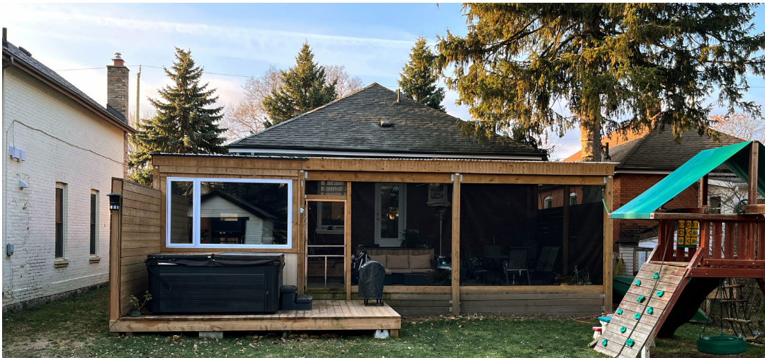
Figure A-1: Progression of the addition in photos, beginning from the top during construction and culminating in completion at the bottom of the page.
