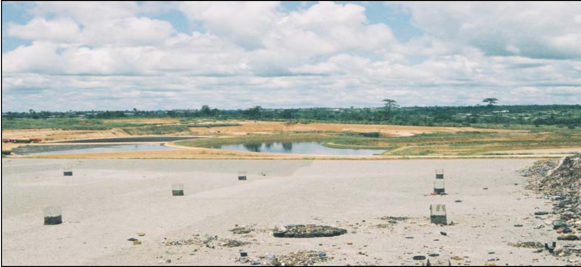
Plate 5-10: Leachate containment and treatment ponds and gas vents at the Kumasi Landfill site
