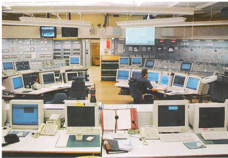
Figure 1: Modernising the Forsmark 3 Boiling Water Reactor Nuclear Power Control Room
