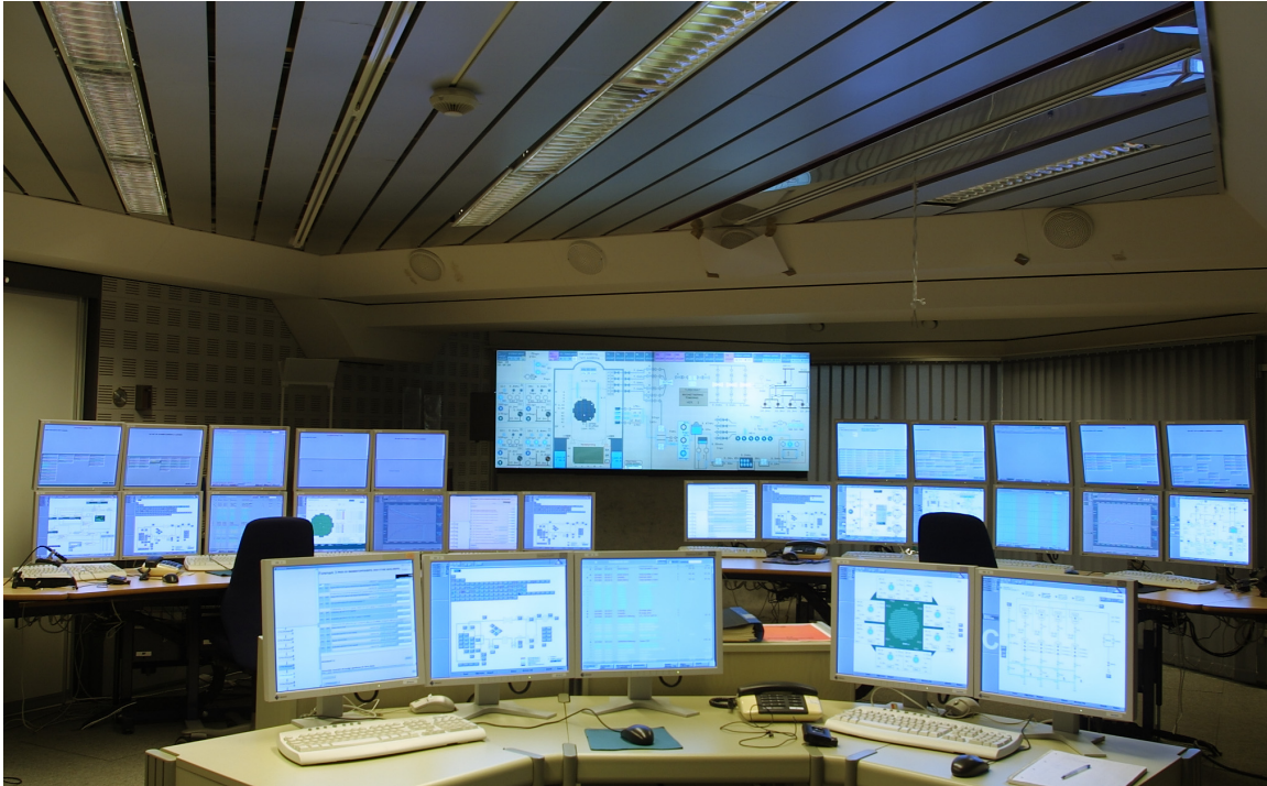
Figure 56: Screen Positioning in Control Room (Skraaning Jr., 2005)
