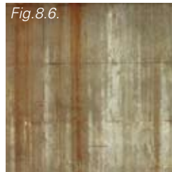
Rust stained concrete
