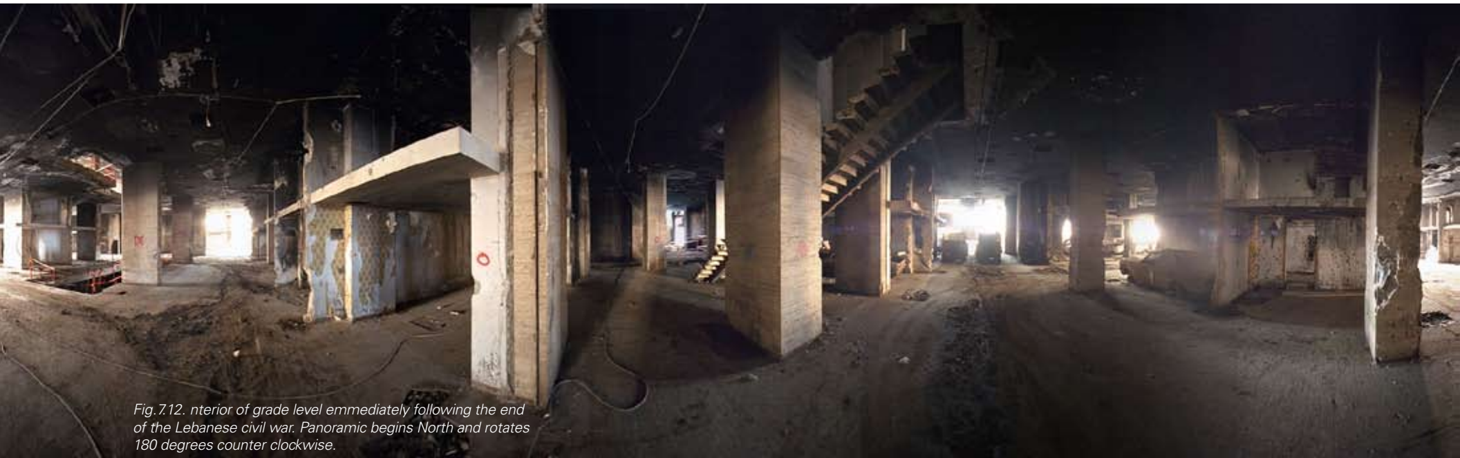
Fig.711. Interior of grade level emmediately following the end of the Lebanese civil war. Panoramic begins North and rotates 180 degrees clockwise.
