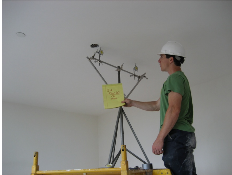
Figure 3-10: Ceiling Deflection Measurement
