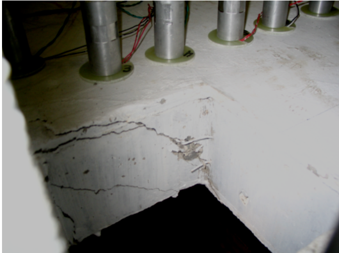
Figure 6.20 - Shear Crack Through Opening, SN6
