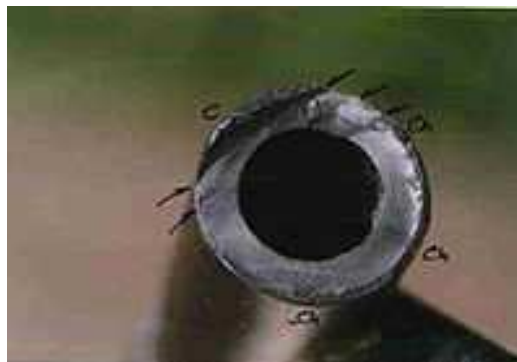
Figure 2.6 Stress Corrosion Cracking [16]
