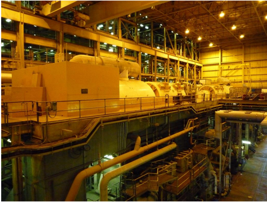
Figure 31 Inside Poplar River Power Station
