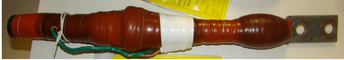
Figure 2.12: Failed cable termination that was connected to 13.8 kV/6.6 kV transformer powering a pump at one of Ontario's nuclear generation station
