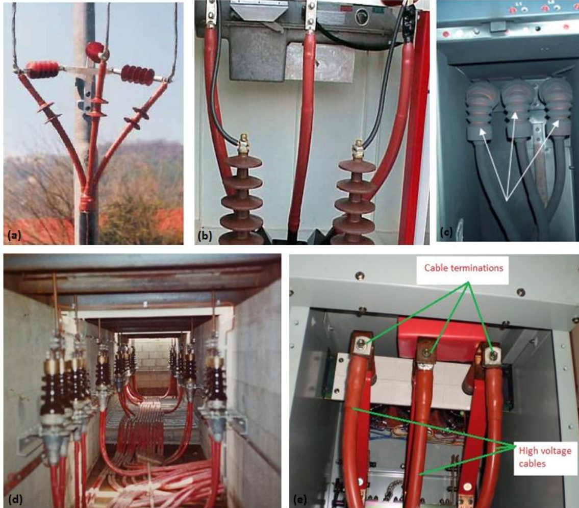
Figure 2.10: MV cable terminations installed at the (a) pole [99], (b) incoming compartment of a harmonic filter bank [99], (c) switchgear [100], (d) substation [101], and (e) electric meter panel [102]
