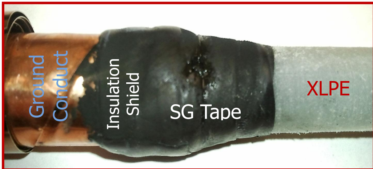
Figure 5.6: Punctured Type-I A at the triple point where the SG tape, XLPE insulation and insulation shield were connected during the PD measurements of Test Case D.
