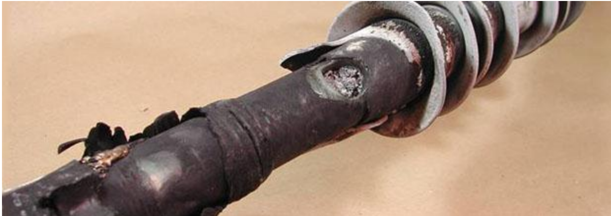
Figure 2.11: Puncture of the 28 kV cable termination located in Ontario due to workmanship error of leaving 2 mm gap at the boundary of stress grading layer and semicon of the cable [103].
