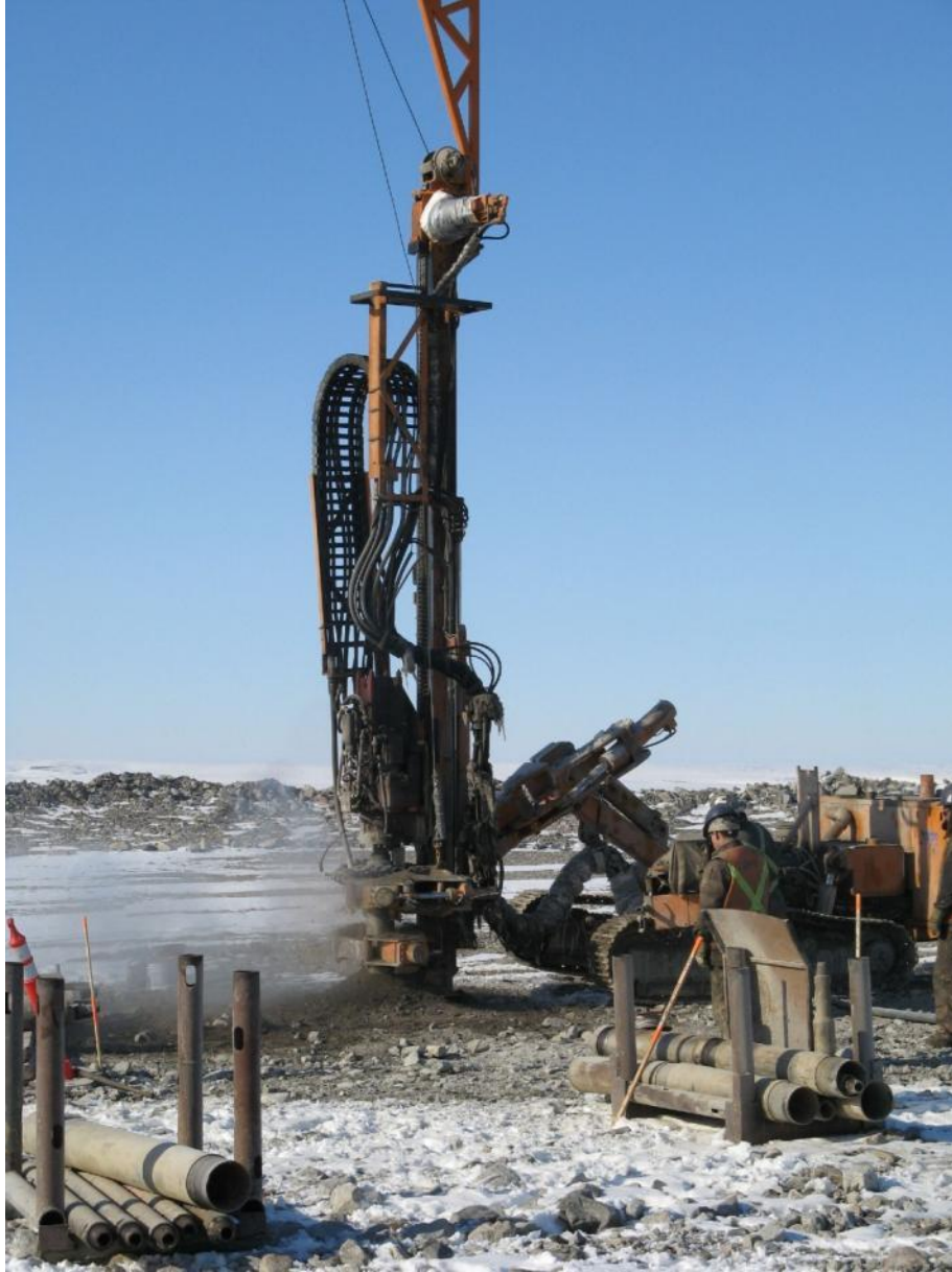
Figure 3-3: Drill hole installation by DNX drilling on the Upper Type III waste rock dump in May 2010.
