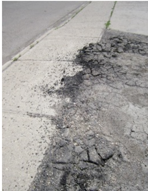
Figure 5-9: Deteriorating Infrastructure in The District
