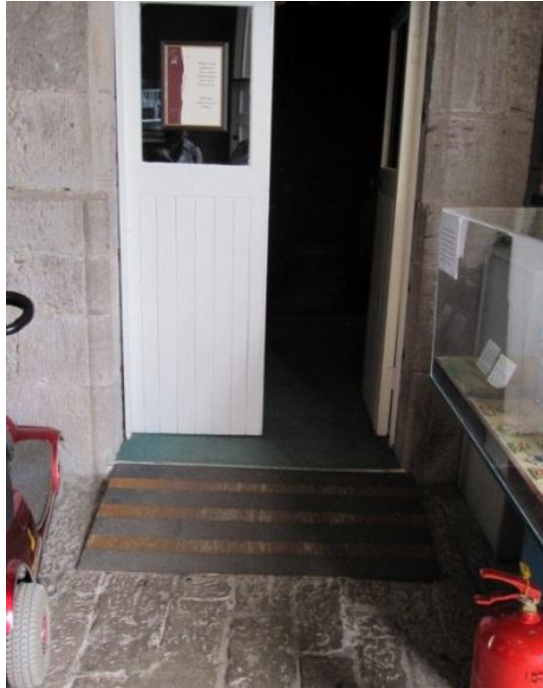
Figure 14. Ramp leading to audio-visual room without space for someone in a wheelchair to easily enter on their own (Barlow, 2011).
