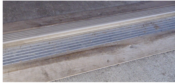
Figure 5.1.1 – The threshold into the doorway was higher than 1.27 cm. To fix the difference in transition over the threshold an angled board is placed on the in/outside of the threshold, which reduces the impact of a poor transition.
