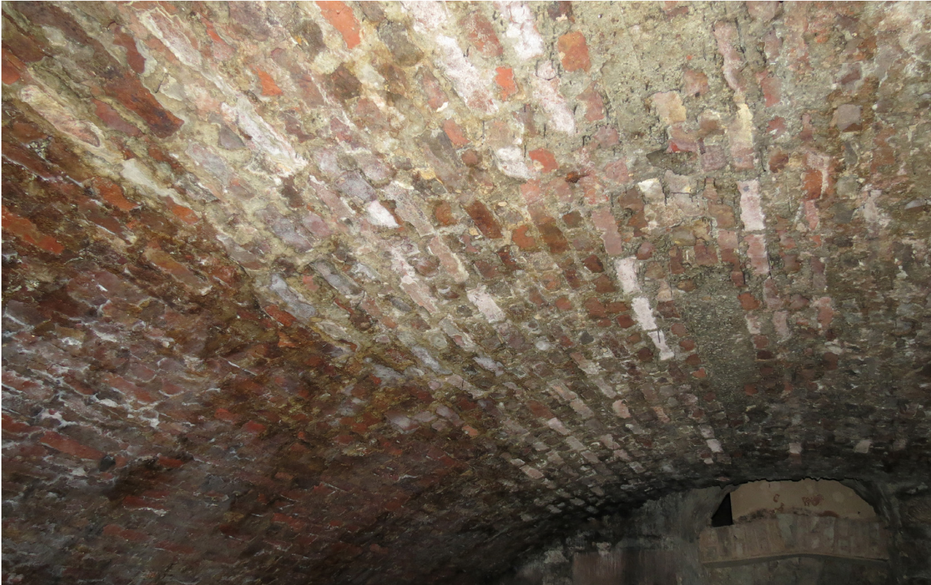
fig. 1.42 | Inside the vaults
