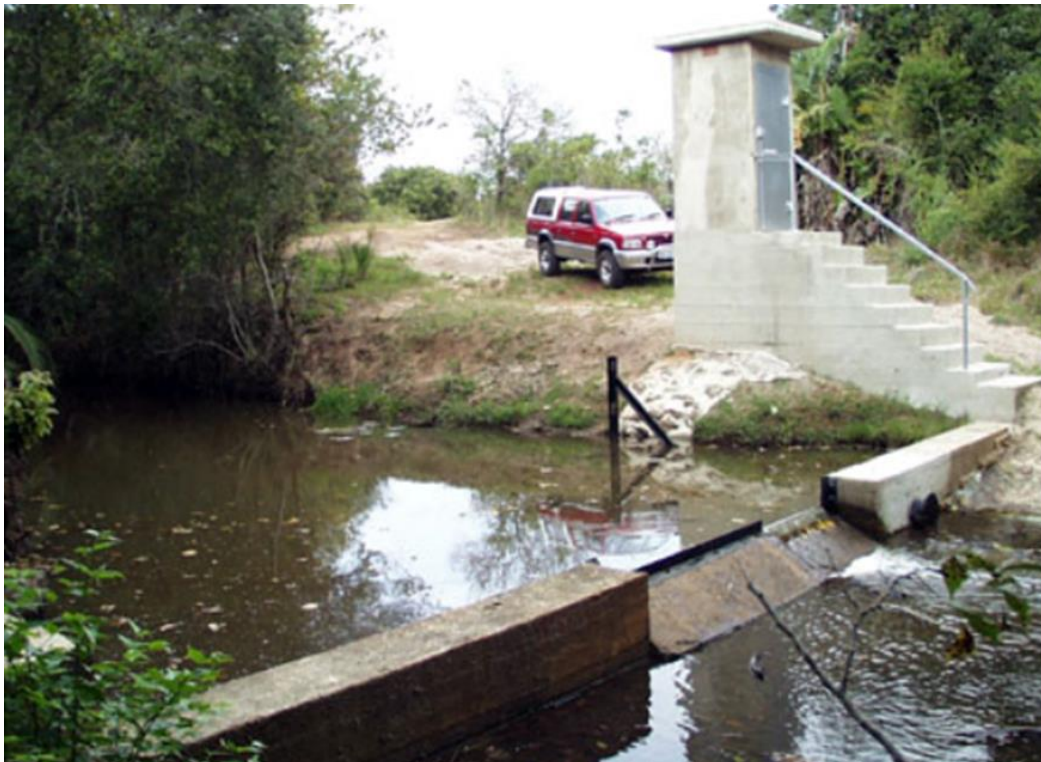
Figure A3: The Mpate stream measuring weir – a rectangular weir (Photo – accessed 22 December 2014: https://www.dwa.gov.za/hydrology/CGI-BIN/HIS/Photos/W3H014.JPG )
