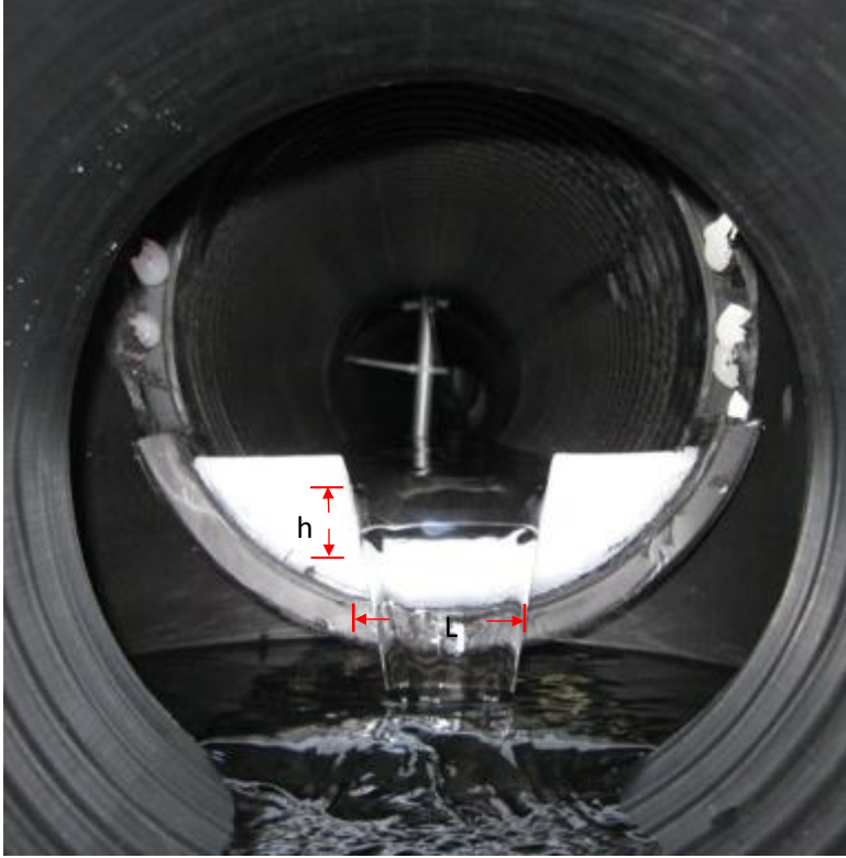
Figure 3-8 Picture of the cipoletti weir from inside the tile (picture taken looking upstream).
