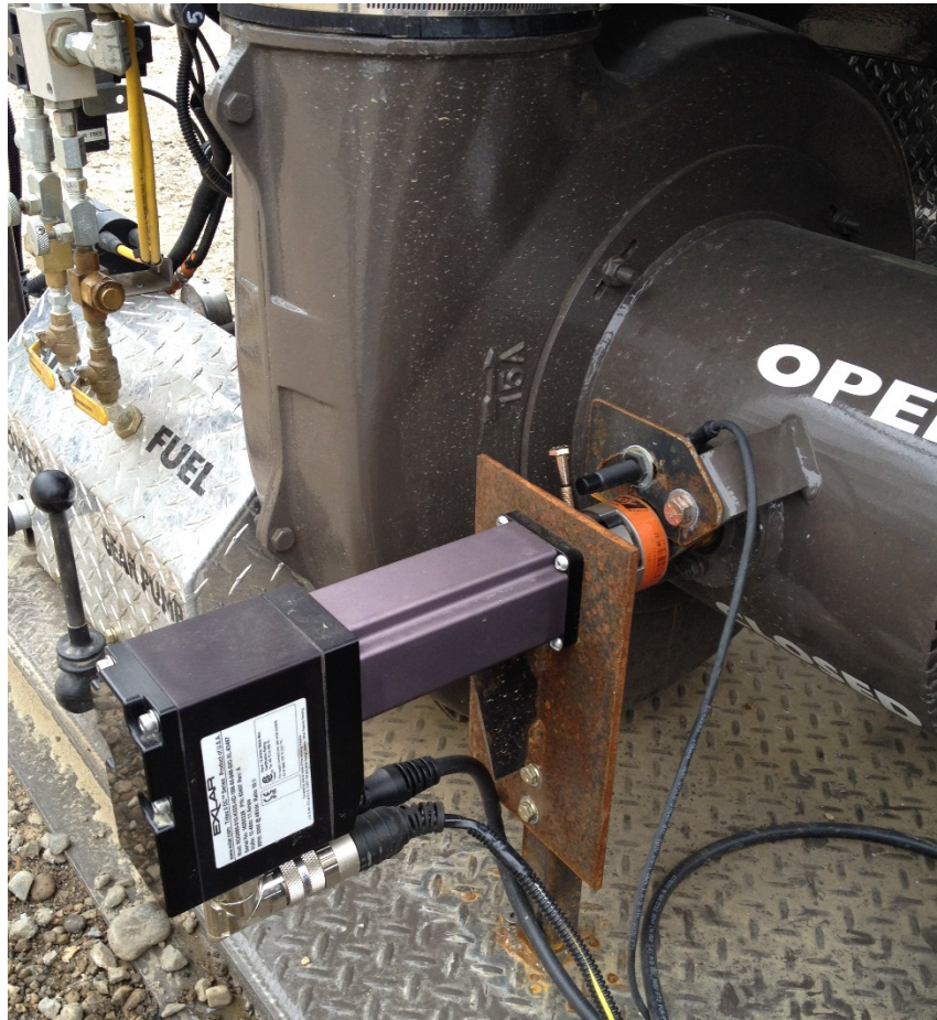
FIGURE 3.10: RDG060 servomotor as installed to control combustion air.
