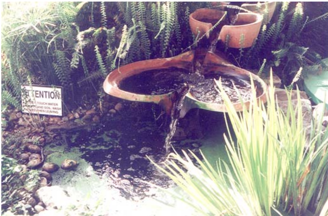
Figure 5-9. Greenhouse-based treatment technology showing Flowform cells and splash pool.
