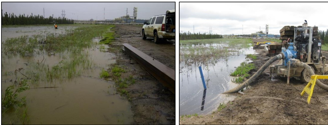
Figure 4-1. Road site flooding photographs June 2013. Left: June 8 and 9 flooding, South view of Pad 106 Access Road. Right: June 11: pumping station installed, water diverted to the drier northwestern side of the road, and flood water migrated down a ditch along Rick George Way to small ponds.
